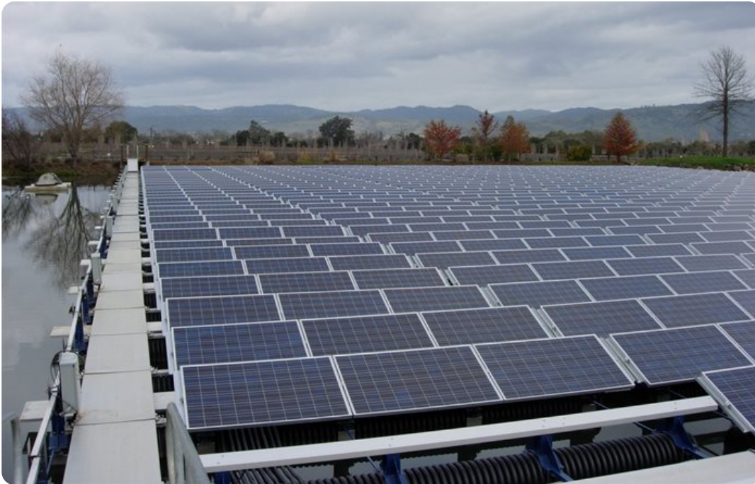
Floating solar system in Napa Valley, California. Source: Wikimedia Commons , CC BY-SA 3.0
